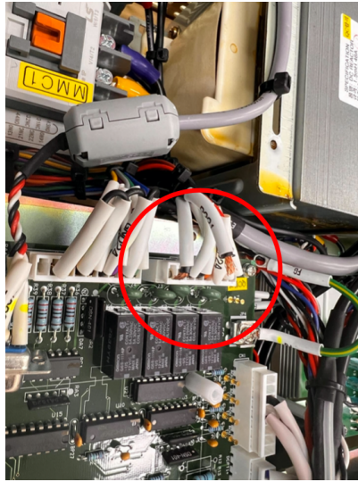
(a) Cable connection 불량
